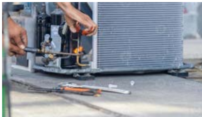
Fig. 5.17: Plumbing and HVAC.
