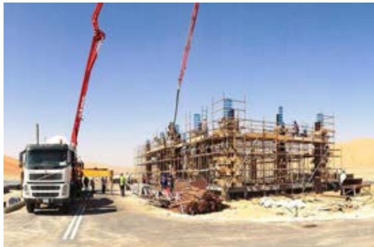
Fig. 6.14: Open space around the work zone to enable fire Service, hoists, and other plants access.
