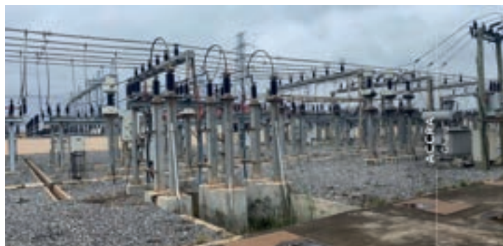
Fig 2.28: Busbars in a Substation
