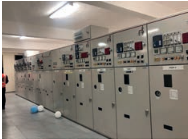
Fig 2.32: Monitoring and Control Panel of a Power Distribution Substation (Source: ECG Station)
