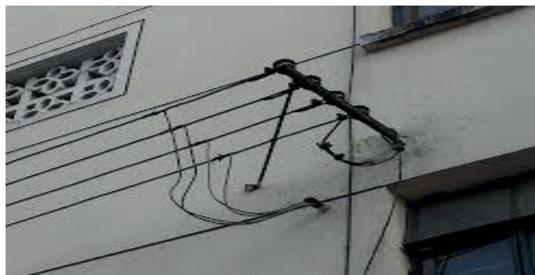
Fig 2.35: Three-phase line connected to a House
