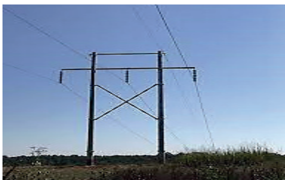
Fig 2.19: Medium Voltage Transmission Line (Source: Medium Voltage Transmission Line - Search Images (bing.com))
