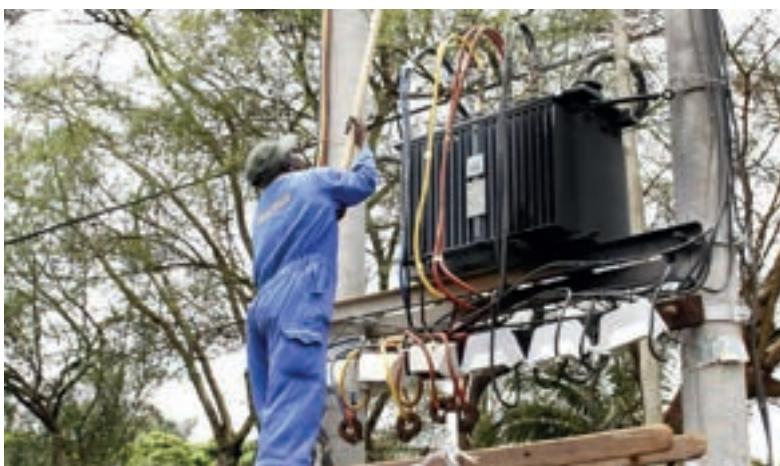
Fig. 3.16: A picture showing a damaged transformer caused by overloaded network.
