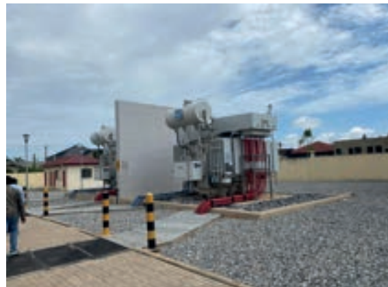
Fig 2.33: Electrical Instrument Transformers (Source: ECG Substation)
