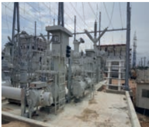
Fig 2.21: High-voltage Distribution Substation
