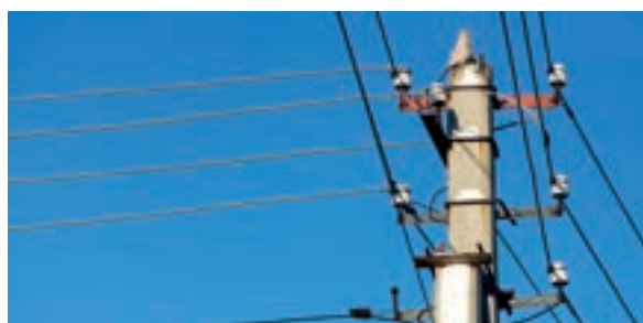
Fig 2.20: Low-voltage Transmission Line
