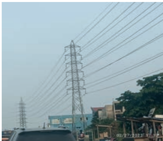
Fig 2.18: High-voltage Transmission Line (33 kV) (Source: ECG Network)
