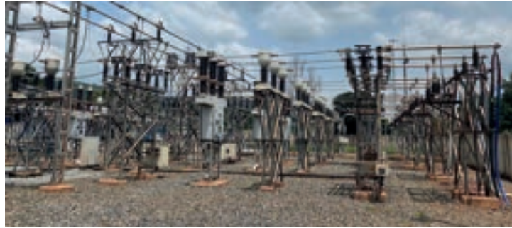
Fig 2.29: Switchgear in a Substation (Source: ECG Substation)
