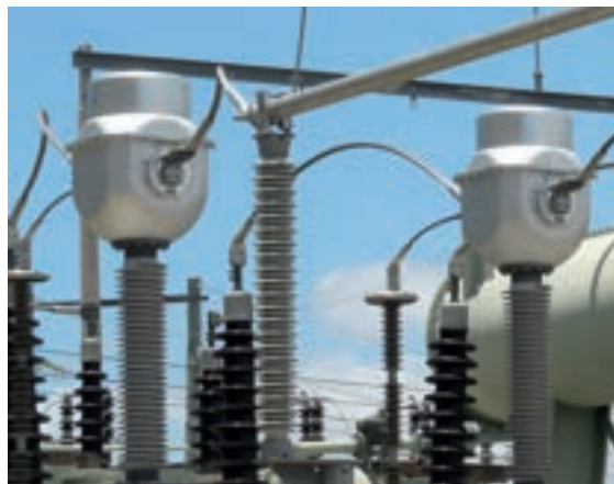
Fig 2.30: Distribution Feeder in a Substation
