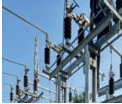
Fig 2.26: Circuit Breakers and Disconnect Switches
