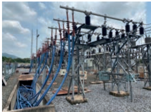
Fig 2.25: Power Lines to a Substation
