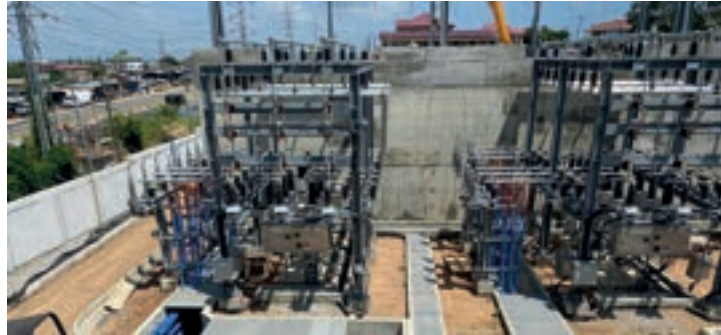
Fig 2.24: Low-voltage Distribution Substation
