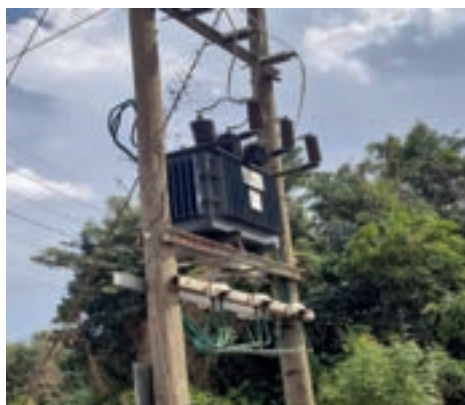
Fig 2.31: Distribution Transformer on a H pole (Source: ECG Station)
