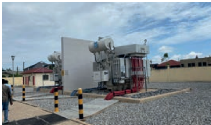
Fig 2.27: Power Transformer in a Substation
