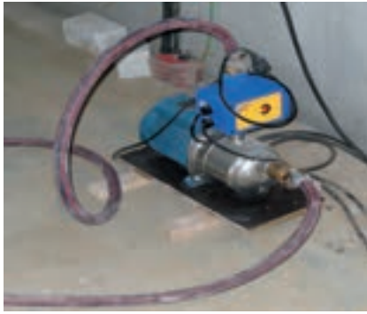
Water pumping machine
