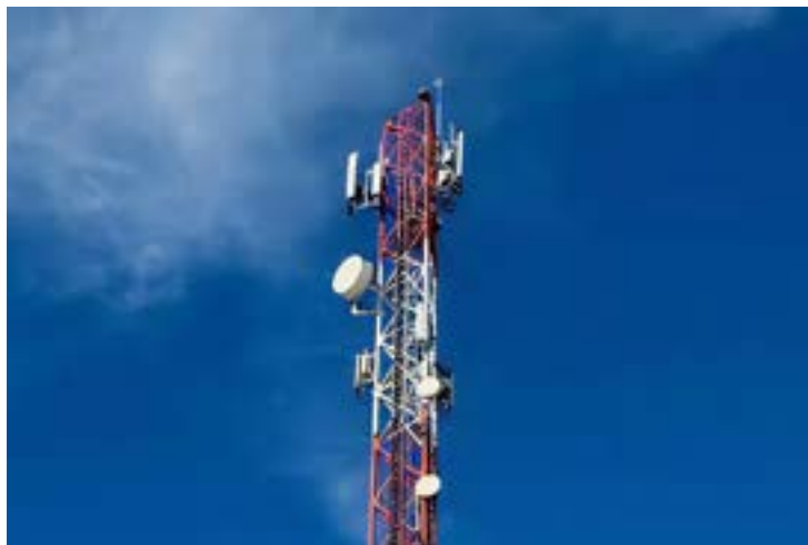
Figure 110: A picture of Telecommunication system
