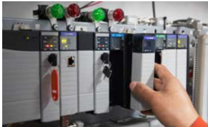
Figure 95: A picture of a PLC
