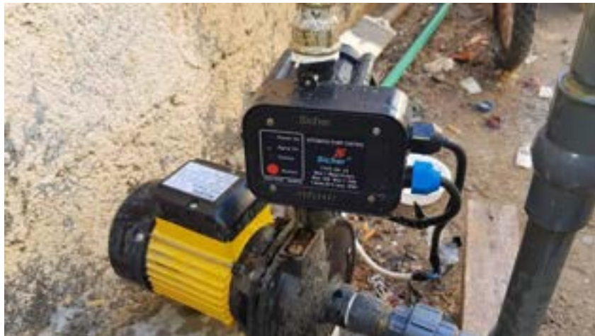
Figure 106: A picture of a Water pump control system
