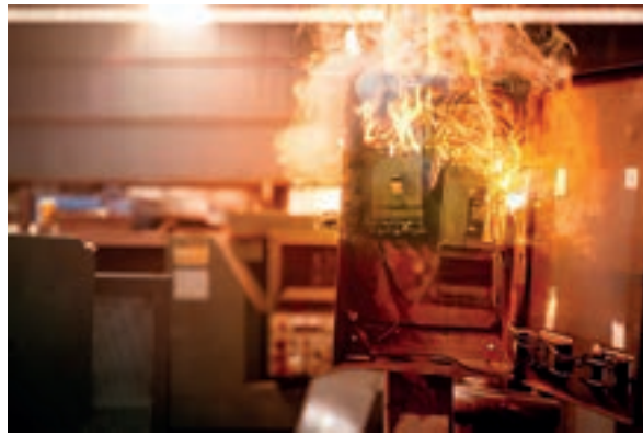
Figure 20: A picture of an electrical accident
