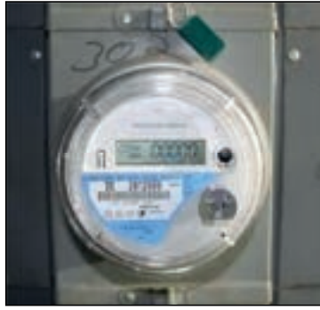
Figure 79: A picture of an Energy meter
