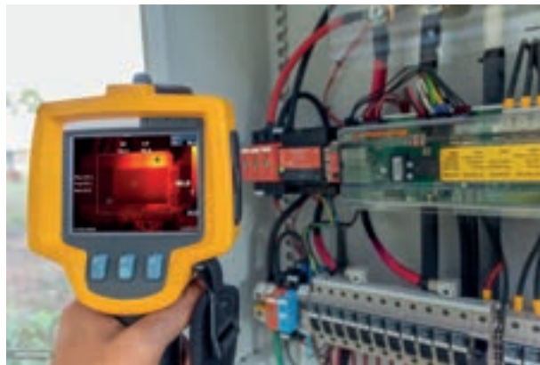
Figure 80: A picture of a Temperature Sensor
