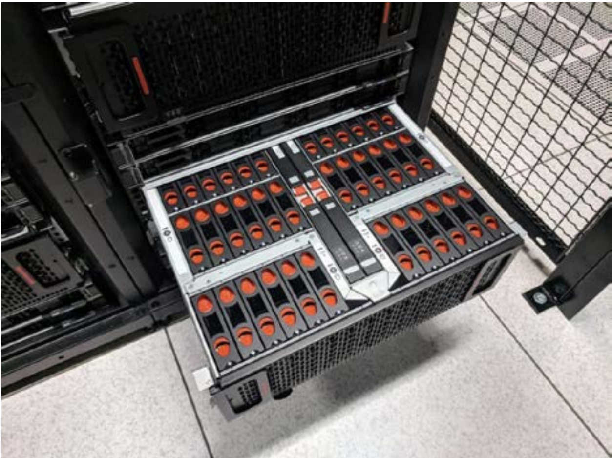
Figure 2.20 SAN showing HDD in RAID to prevent data loss.
