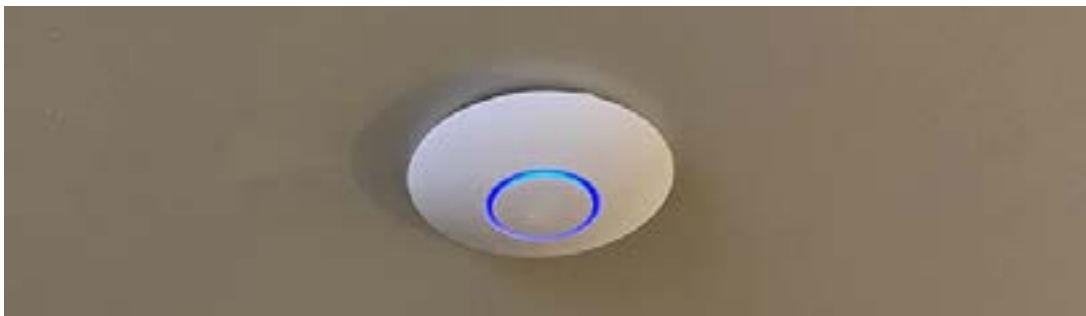
Figure 2.26 Wireless Access Point fixed on a ceiling.
