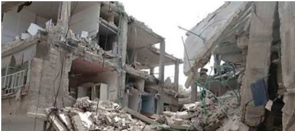
Fig. 2.1: A picture of a structural failure
