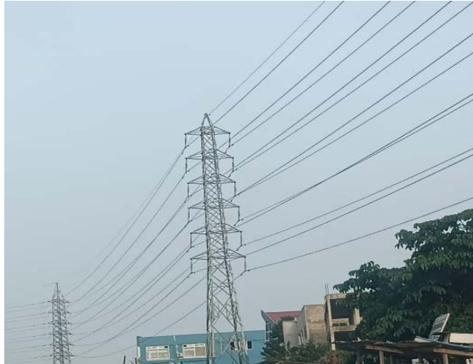
Fig 2.4.6: High-voltage Transmission Line (33 kV)
