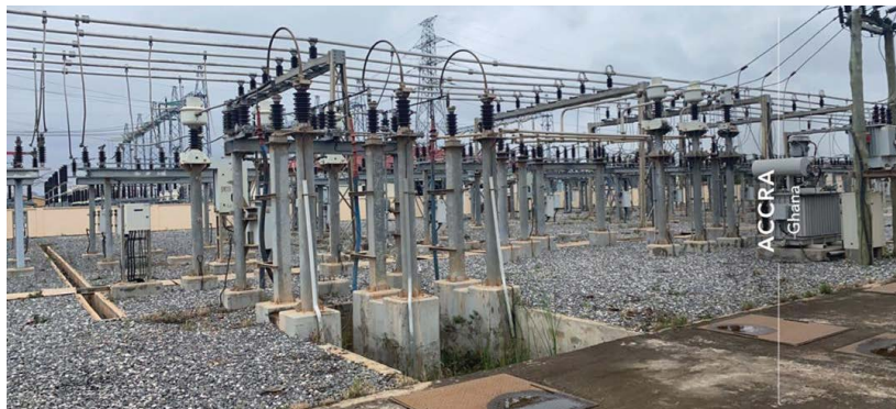
Fig 2.4.16: Busbars in a Substation
