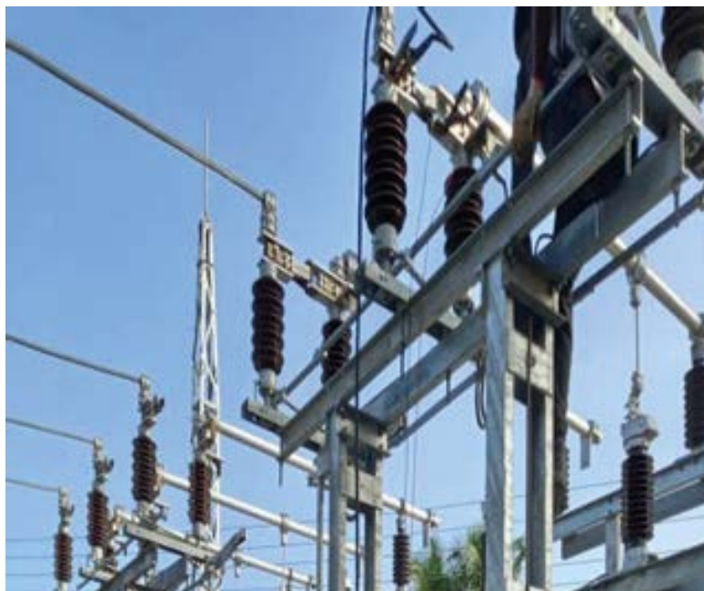
Fig 2.4.14: Circuit Breakers and Disconnect Switches
