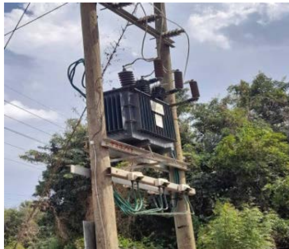
Fig 2.4.19: Distribution Transformers on a H pole
