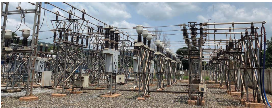
Fig 2.4.17: Switchgear in a Substation
