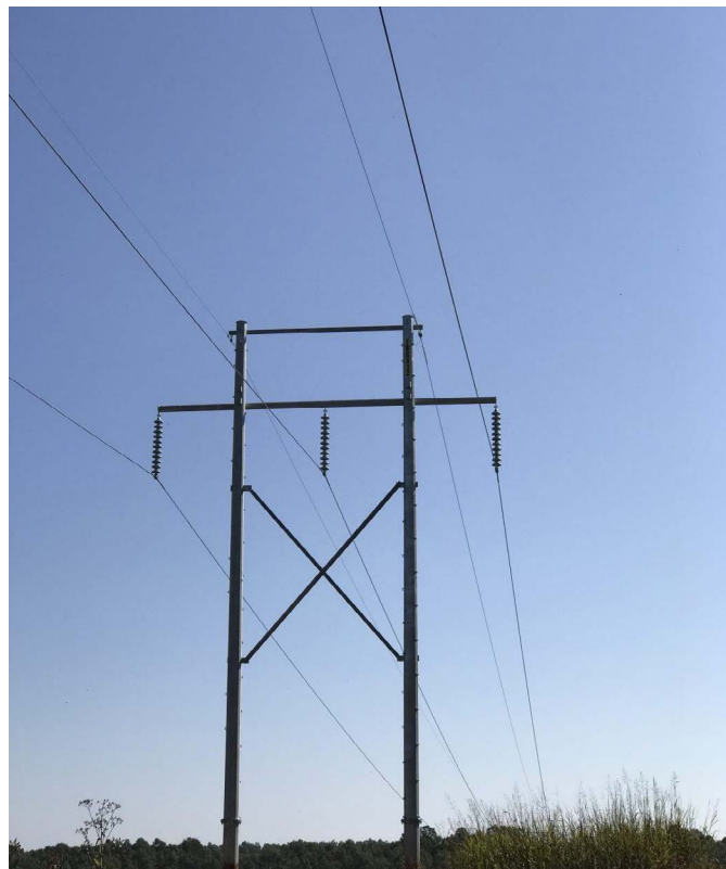
Fig 2.4.7: Medium Voltage Transmission Line
