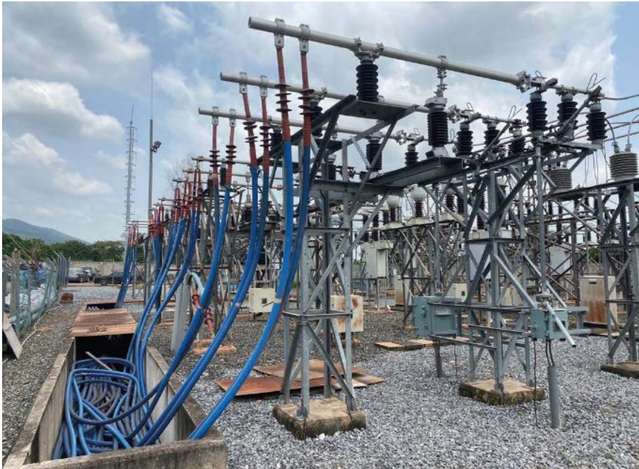
Fig 2.4.13: Power lines to a Substation
