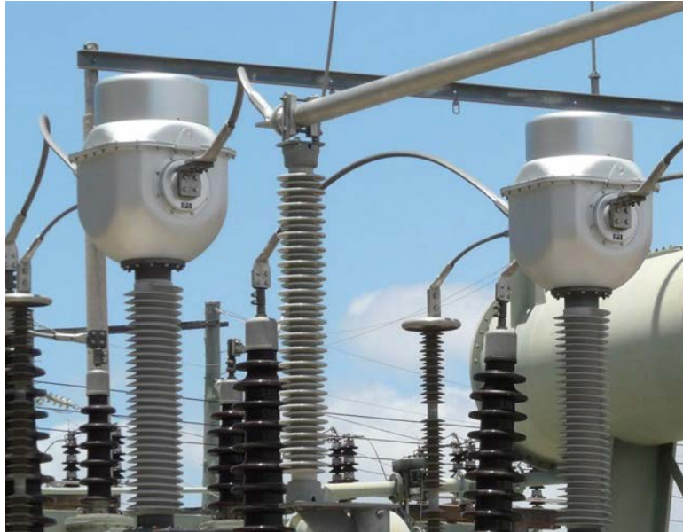
Fig 2.4.18: Distribution Feeder in a Substation
