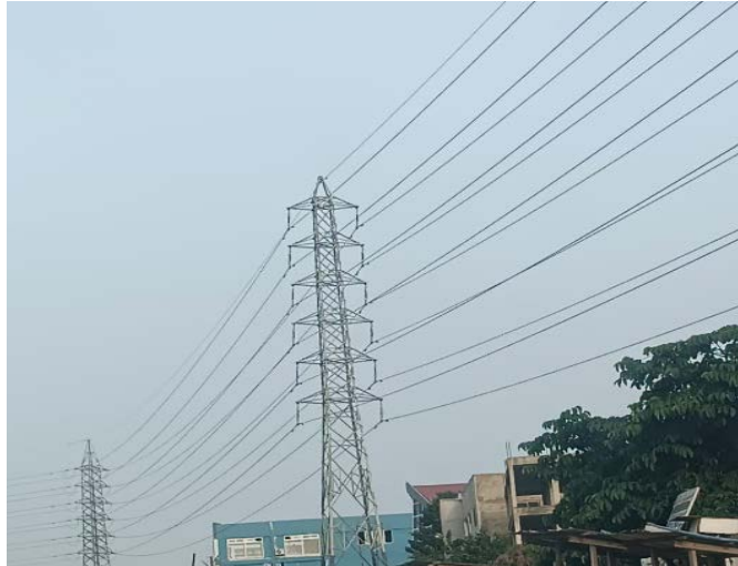
Fig 2.4.6: High-voltage Transmission Line (33 kV)
