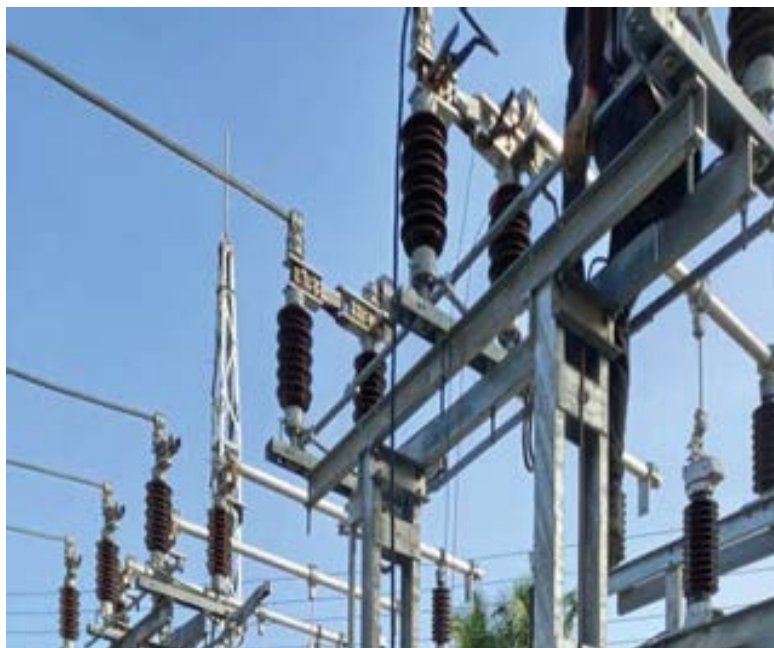
Fig 2.4.14: Circuit Breakers and Disconnect Switches
