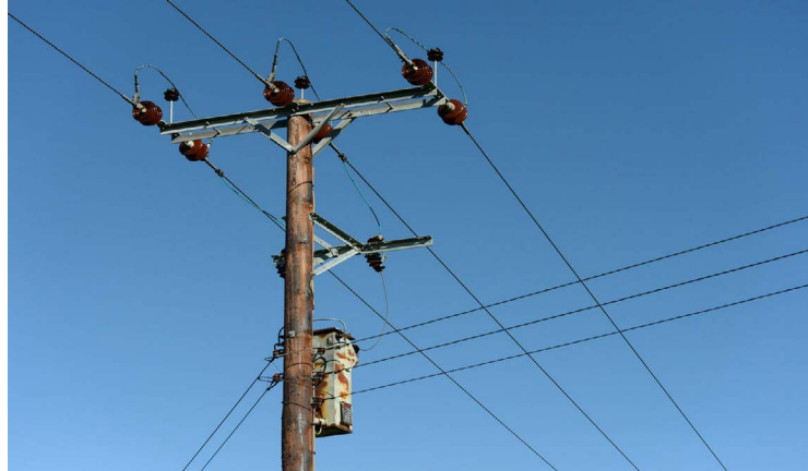
Fig 2.4.8: Low-voltage Transmission Line
