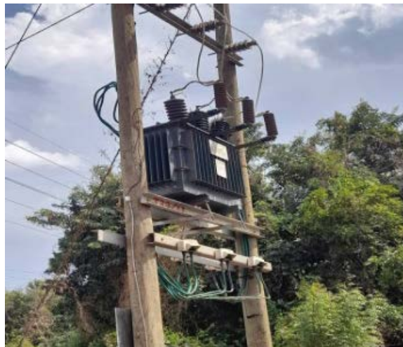
Fig 2.4.19: Distribution Transformers on a H pole
