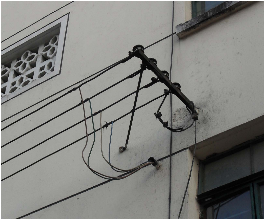
Fig 2.4.22: Three-phase distribution line
