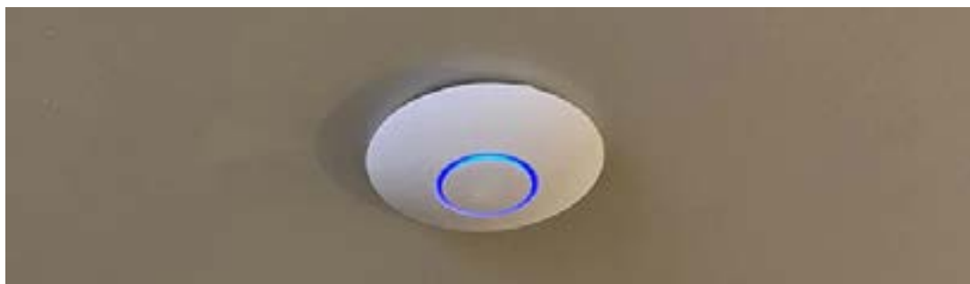
Figure 2.26 Wireless Access Point fixed on a ceiling.
