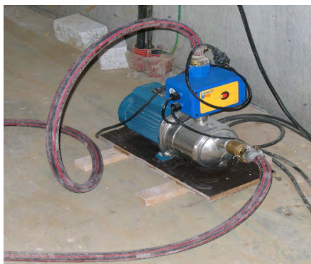
Figure 2.1: A water pumping machine
