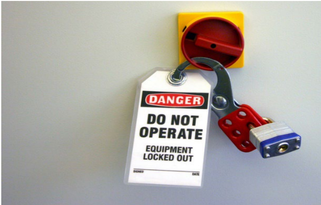
Fig. 3.2.12: A lockout being applied to a device
