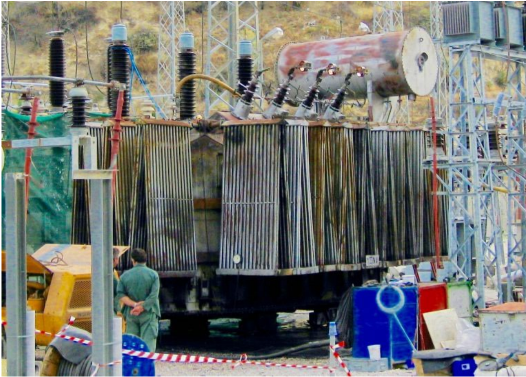
Fig.3.4.2: Picture of a damaged transformer (bing.com.)
