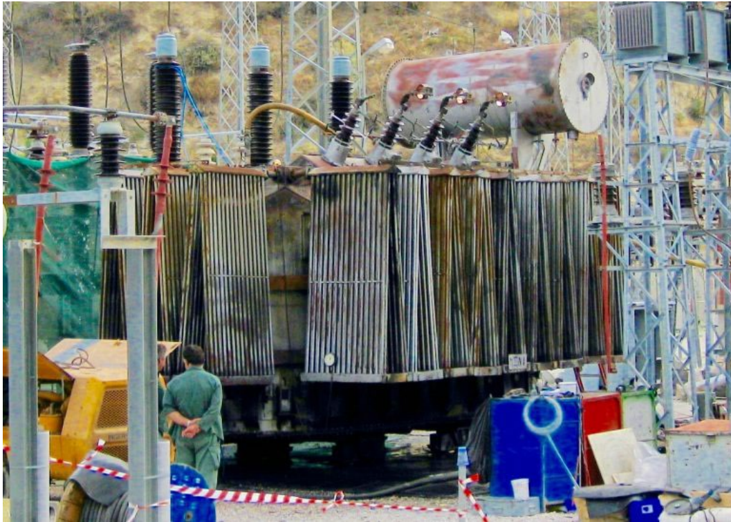
Fig.3.4.2: Picture of a damaged transformer (bing.com.)
