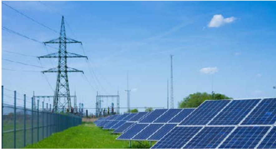
Fig. 5.1: A picture of a Solar Generation Station
