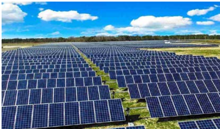
Fig. 5.12: A picture of solar panel
