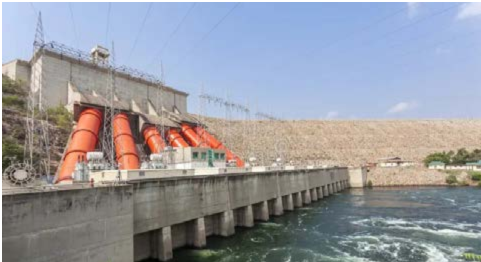
Fig. 5.3: A picture of a Hydro Energy Generation Station
