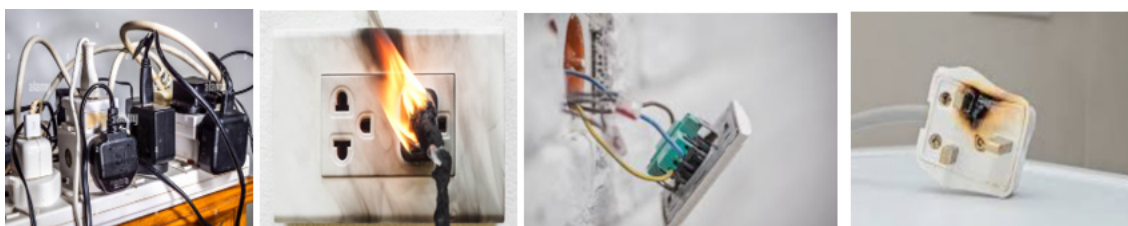
Figure 5.14: Overloaded and Faulty Sockets
