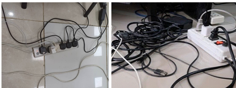
Figure 5.13: Cables and Cords running across floors
