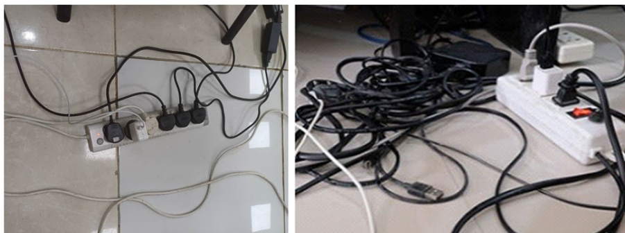
Figure 5.13: Cables and Cords running across floors
