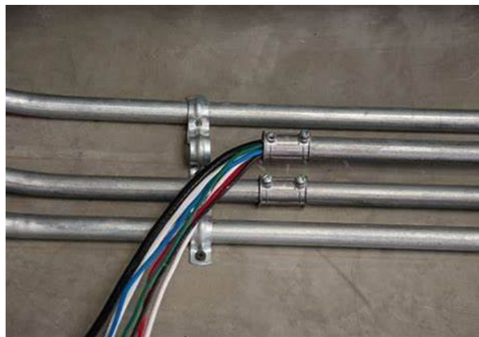
Figure 2.4: A picture of surface conduit wiring
