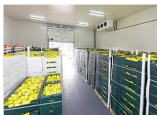
Cold Storage Unit
