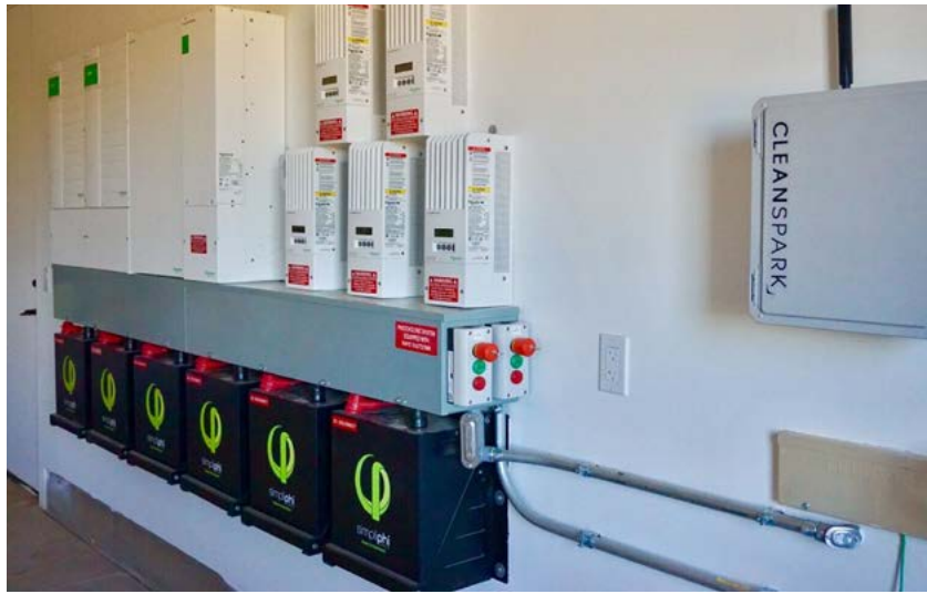
Figure 5.4: A picture of Photovoltaic batteries
