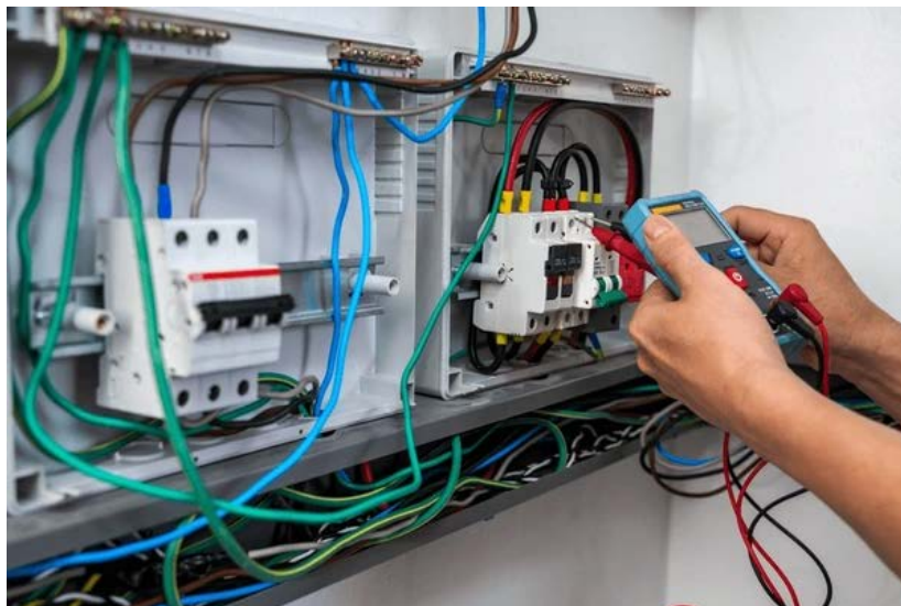
Figure 5.5: A picture of circuit breakers in combiner boxes
