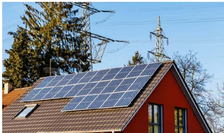
Figure 5.2: A picture of Photovoltaic Modules on a roof
