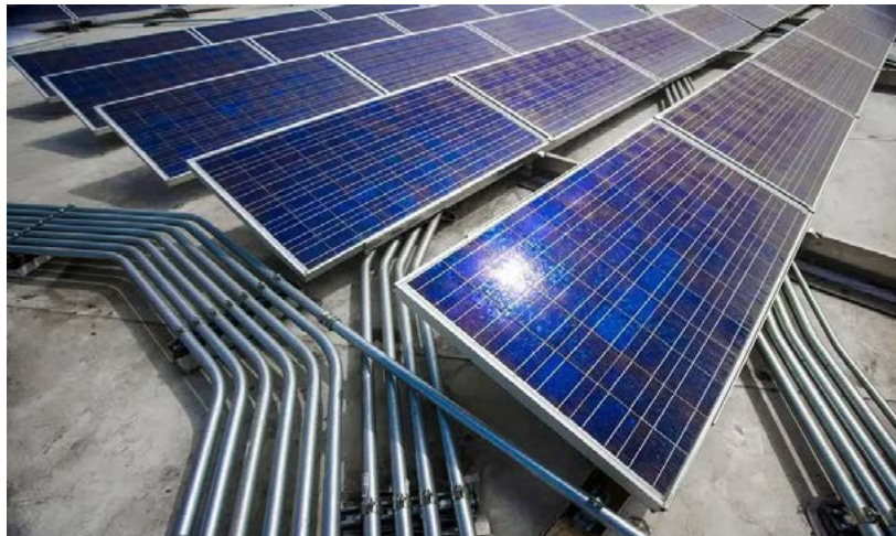
Figure 5.7: A picture of photovoltaic wiring
