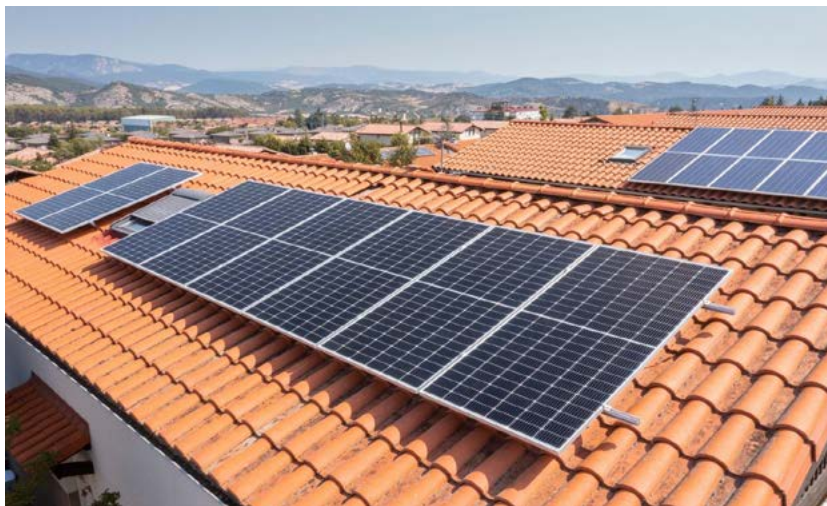
Figure 5.9: A picture of solar collectors on rooftop
