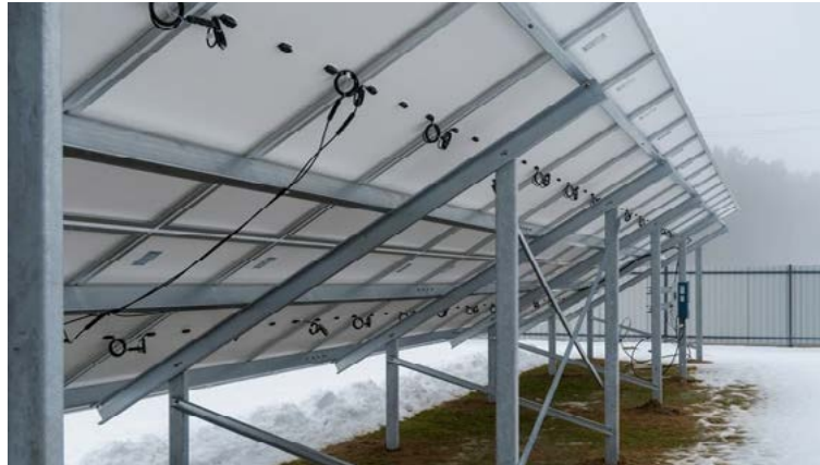
Figure 5.2: A picture of the PV module mounting system
