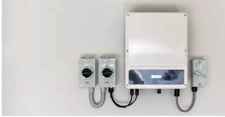
Figure 5.1: A picture of an inverter connected to a PV module
