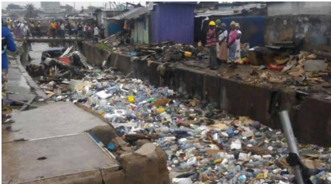
Figure 9.1: Chocked gutter likely to cause flood
