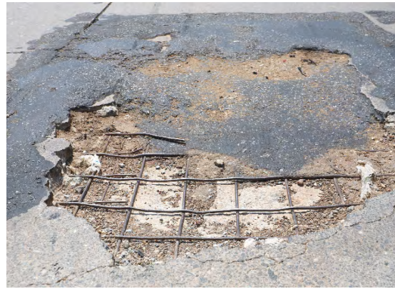
Image 2 (most part deteriorating now)
