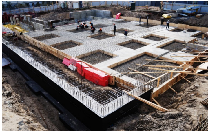
Figure 2.24: Foundation concrete having direct contact with the ground
