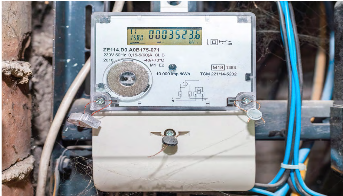
Fig. 13.5: Digital electric meter
