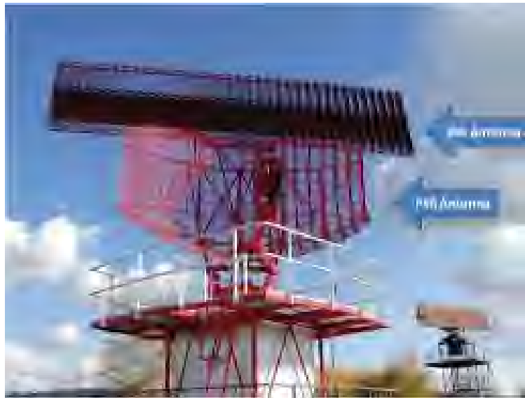
Figure 3.15: PSR/SSR antenna system
