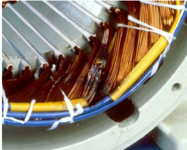
Figure 3.10.3: Failure in a three-phase stator winding of an electrical motor.
