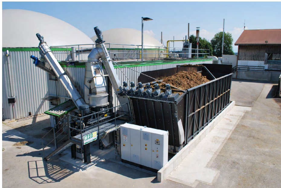
Figure 5.11: Picture of the Feeding Mechanism of a Bioenergy system
