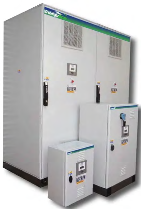
Figure 6.14: Picture of Power Factor Correction Device
