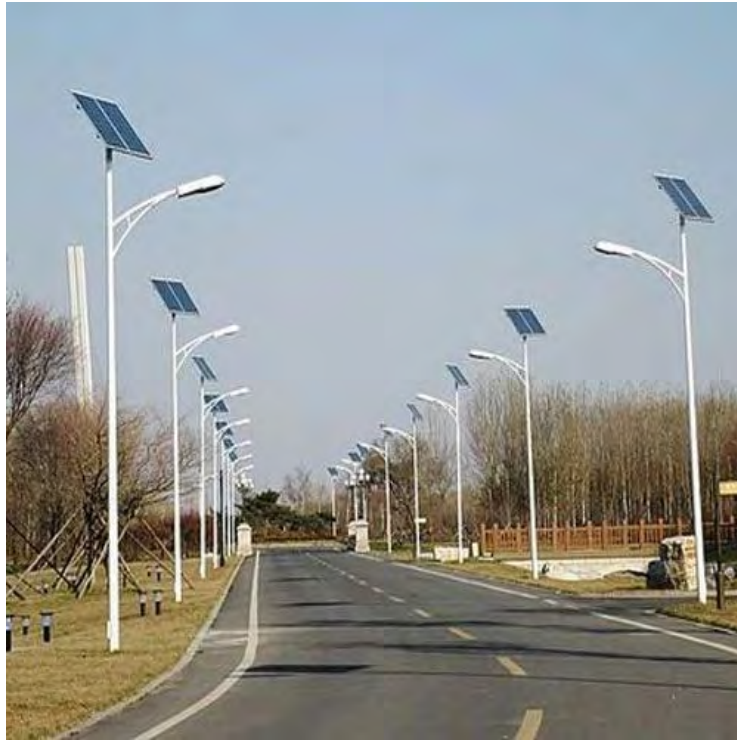
Figure 6.11: Picture of Solar Outdoor Lighting
