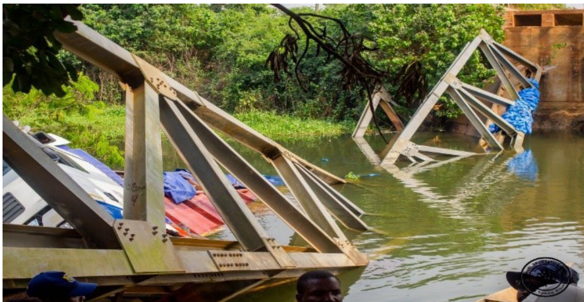
Figure 2.16: Collapse of bridge linking Adidome, Juapong leaving residents stranded (Aggor, 2024) https://citinewsroom.com/2024/01/collapse-of-bridge-linking-adidome-juapong-leaves-residents-stranded/
