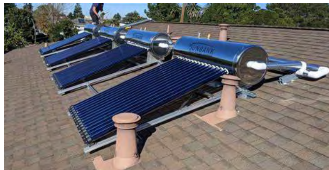
Figure 33: Solar Water Heaters
