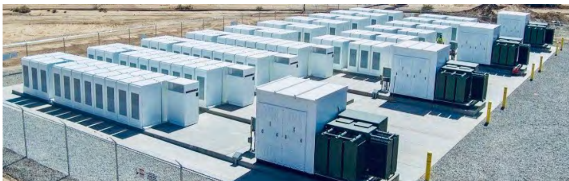
Figure 17: Bioenergy Storage System
